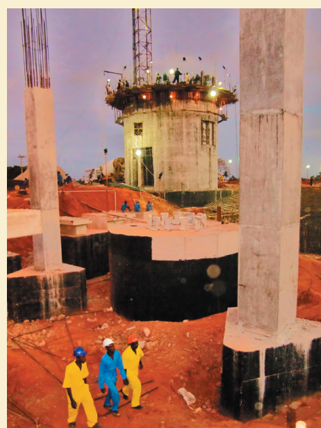
Dar Es Salaam Cement Grinding Plant, with a capacity of 750,000 tons per year, under construction. The Plant is scheduled for commissioning in December 2011.
